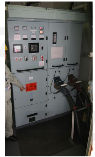
Container vessel connection point on-board
