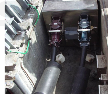
Container vessel connection box at shore
