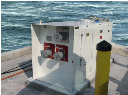
(3) 200A Russellstoll Modules Color coded for vessel connection
