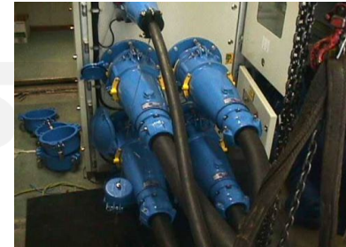
Cruise vessel connection point on-board vessel
