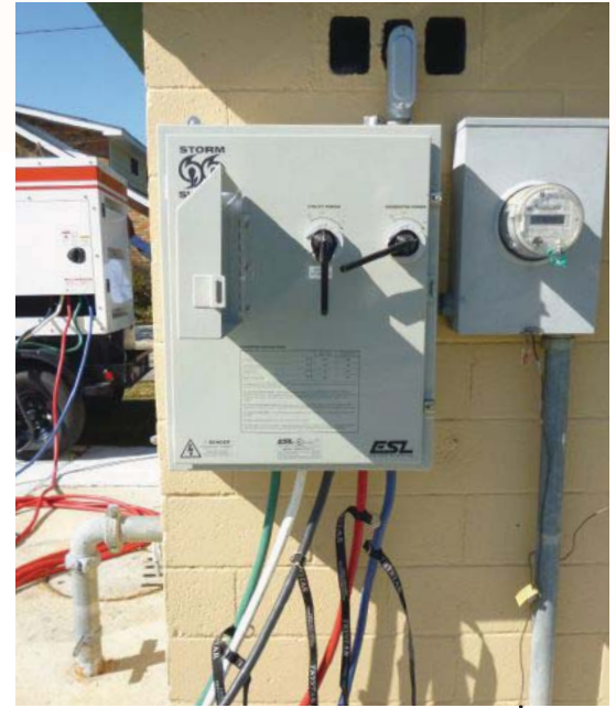
Figure 2: With the help of a portable generator, this MTS provides emergency backup power to a business.
