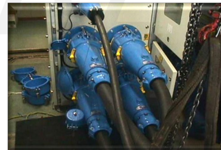
Cruise vessel connection point on-board vessel
