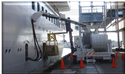
Shore based mobile cable management system
