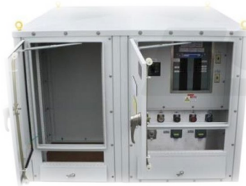
Broadcast Truck Power Pedestal
